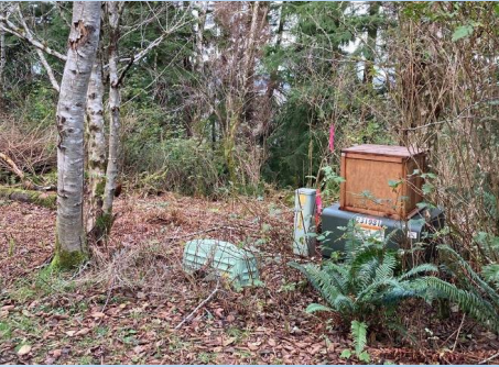
Transformers & pedestals can be found throughout the undeveloped areas
