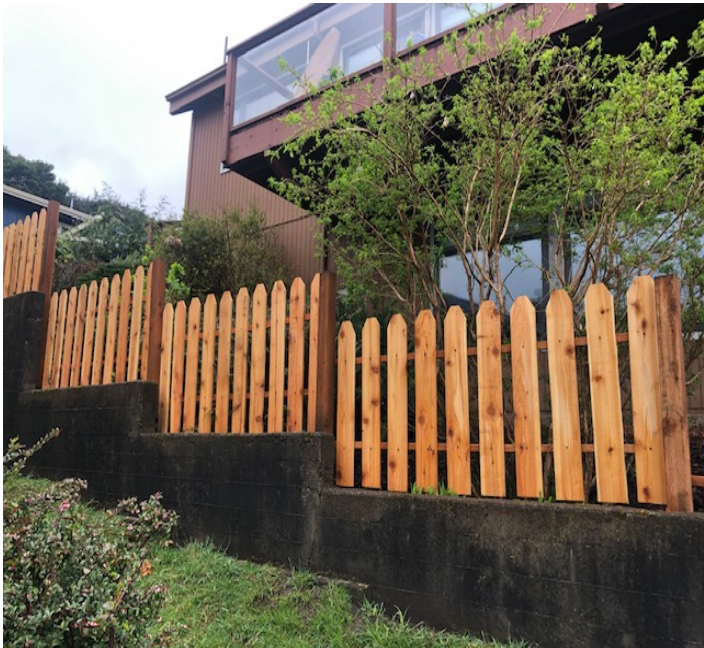
View from north side pre-repair—circa June 2020
